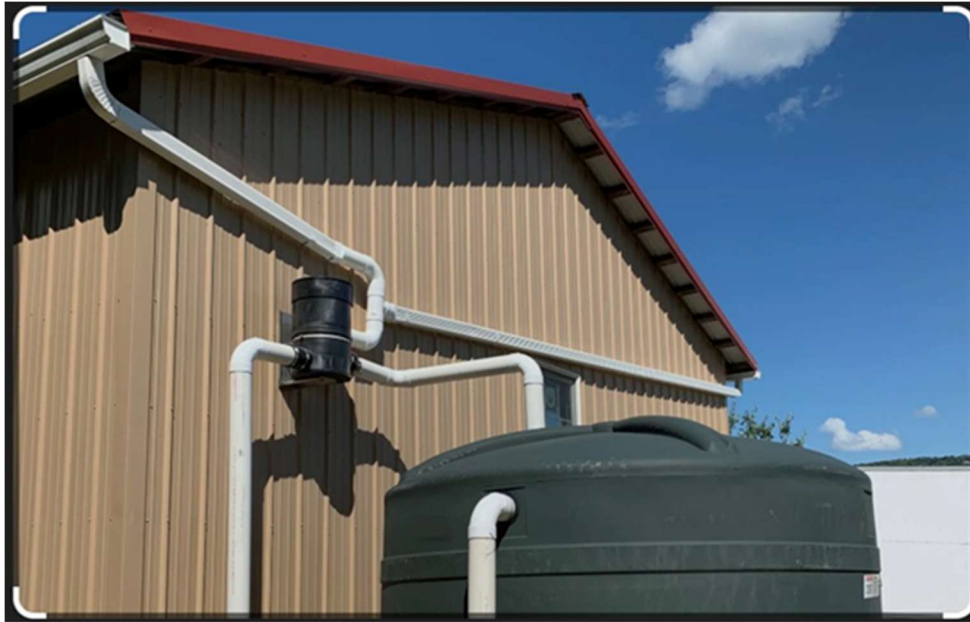
Figure 13.1: Rainwater Storage Unit
